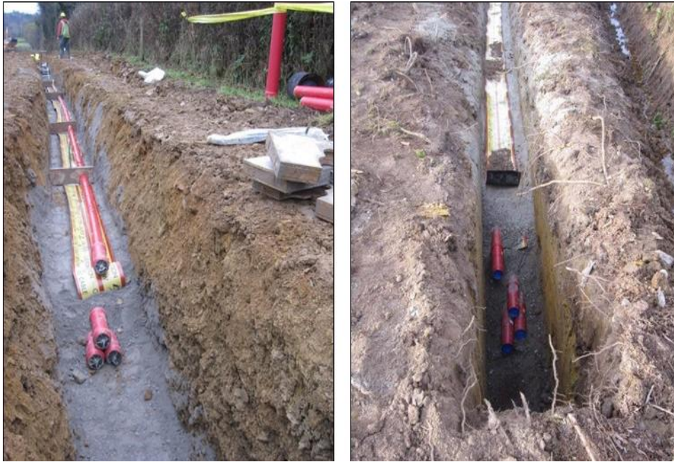
Plate 2-2 Typical Trefoil Cable Trench View
